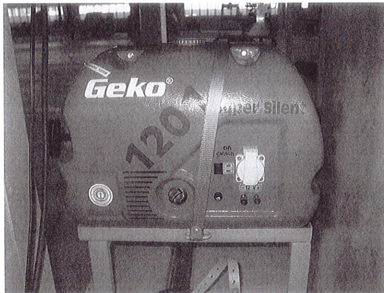
Picture 7: Portable Generator Set
